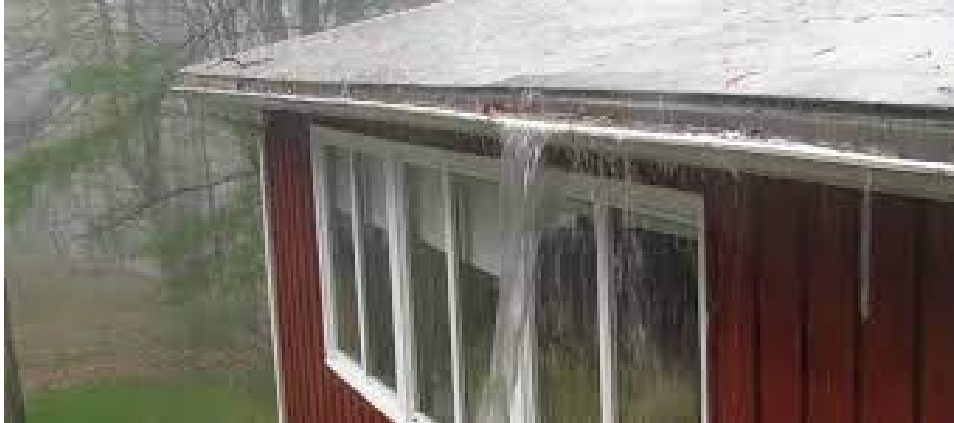
Inadequate Gutters Size
